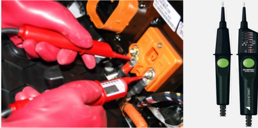
Figure 8: Checking for Absence of Voltage with a Voltage Tester
