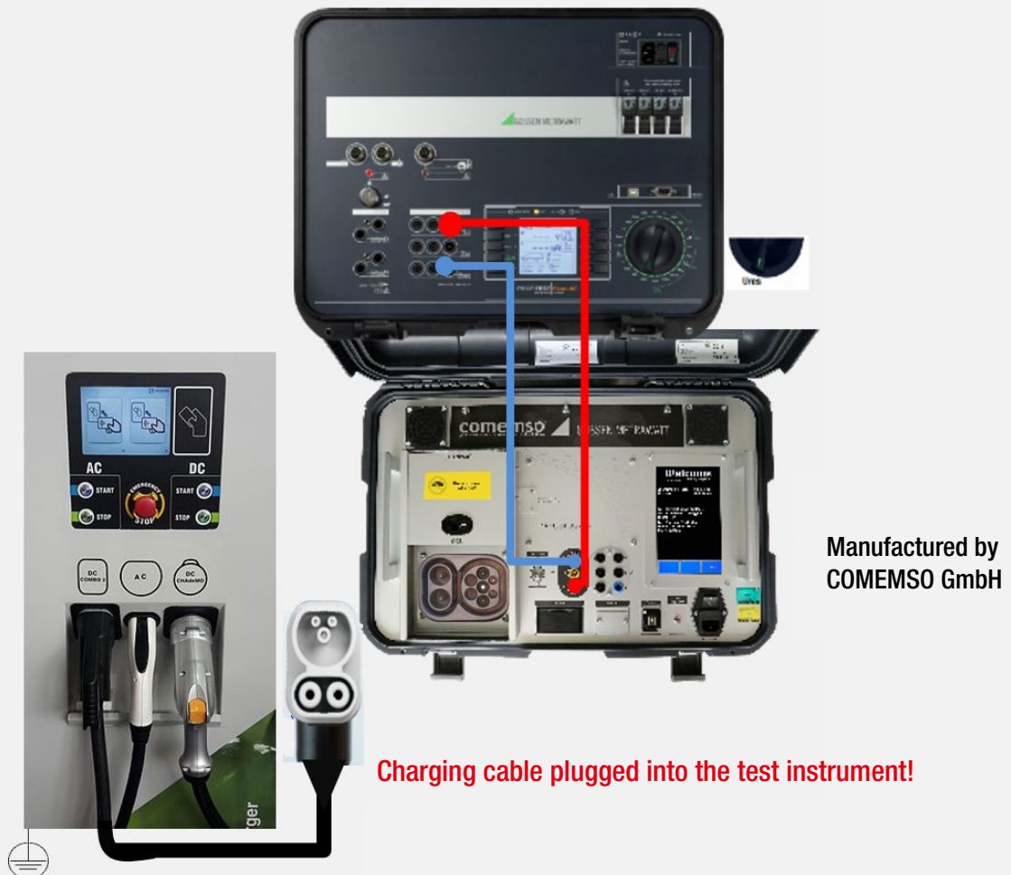
Figure 3: Test Setup at DC Charging Station with PROFiTEST H+E XTRA C and PROFiTEST PRIME
